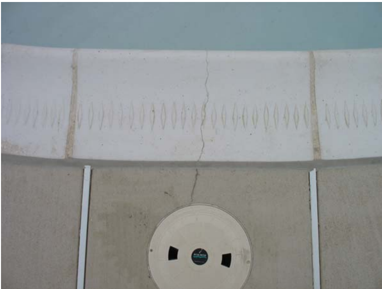
Photo 15 – Cracked coping at southeast corner of wading pool.
