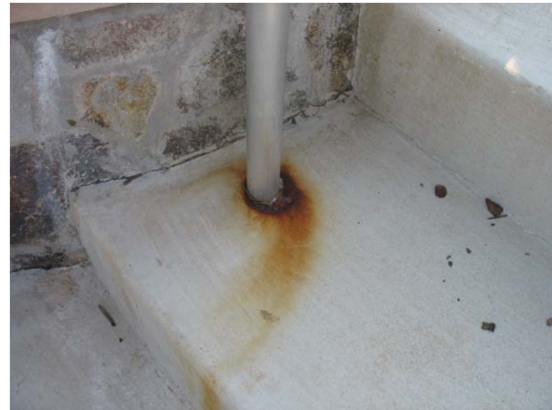
Photo 8 – Rust forming on handrail base at club house entry stairs.
