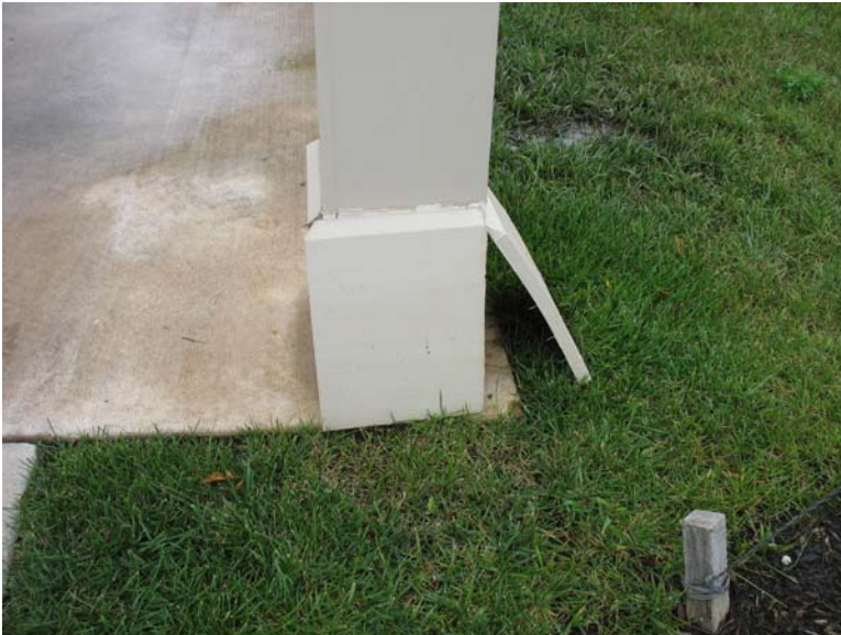
Photo 5 – Damaged wood trim at pool entry gazebo.
