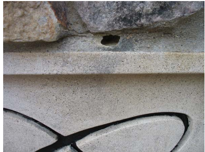
Photo 16 – Hole in mortar above “G” at Glenkirk Road entry sign.
