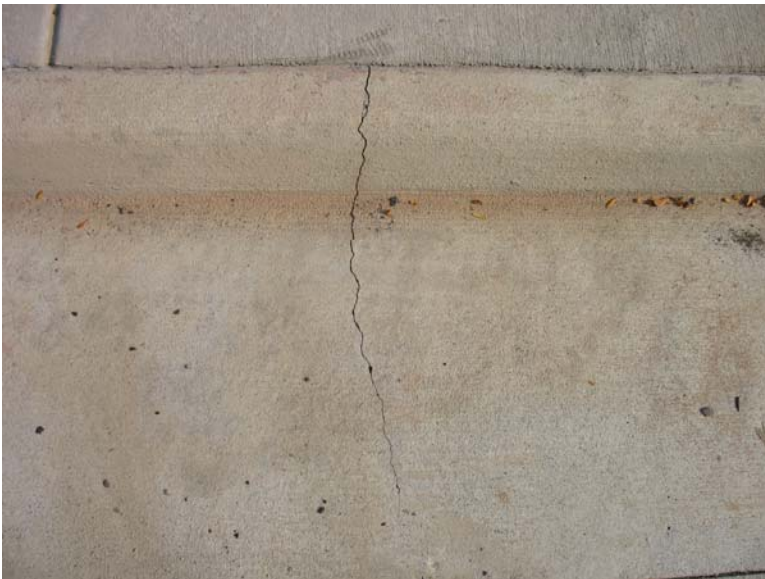
Photo 3 – Cracked curb and gutter at pool parking lot, SW corner.
