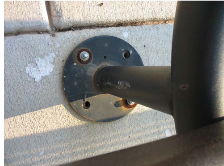
Photo 10 – Two missing bolts on park bench post near pool.
