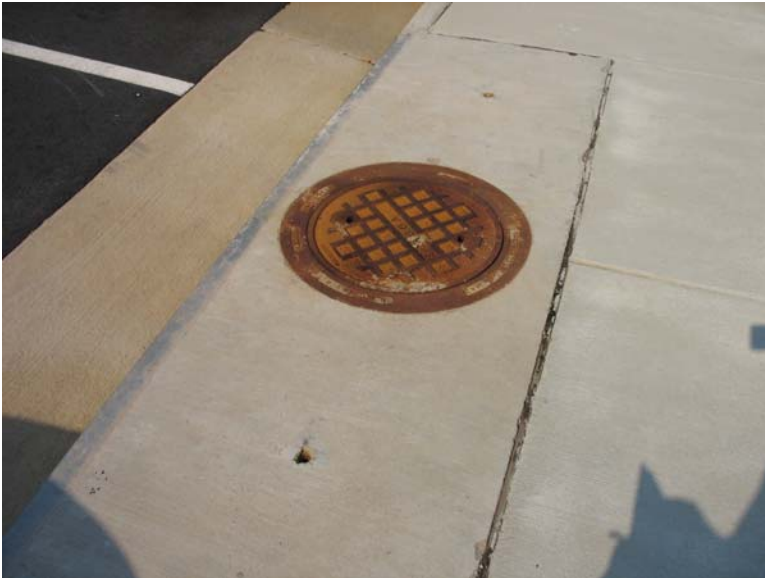
Photo 1 – Holes in concrete at storm sewer inlet, pool parking lot.
