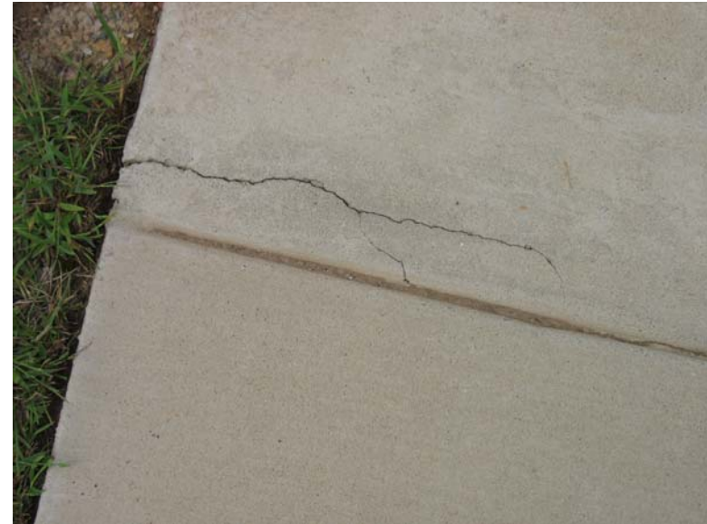
Photo 2 – Cracked sidewalk section adjacent to 8724 Lords View Lp.
