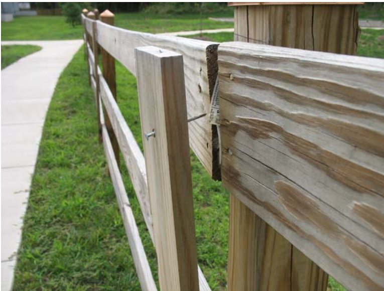
Photo 7 – Loose fascia trim on guardrail behind 8720 Lords View Lp.
