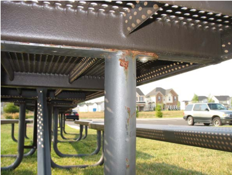
Photo 9 – Rust forming on picnic table post near pool area.
