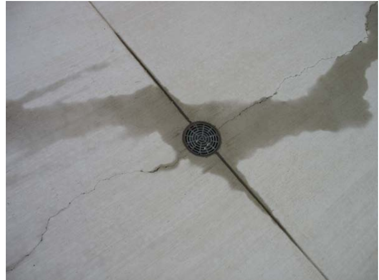
Photo 14 – Cracked pool deck at south end of the main pool.
