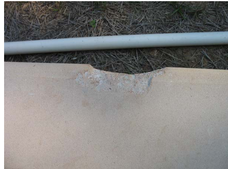
Photo 4 – Broken wall cap at entry feature south of Rollins Ford Rd.
