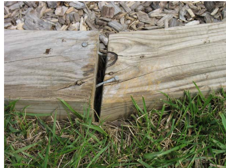
Photo 12 – Exposed nail on playground timber behind 8676 Wales Ct.
